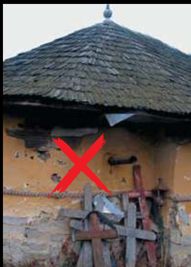
Improper stove chimney piercing the wall.
