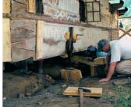
Elevation of the church to replace bottom logs and build a stone foundation in 2013.
