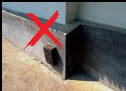
The stone base has been covered in concrete all along the church outline and will deteriorate the wood.
