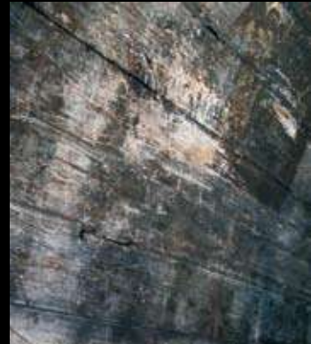
Example of painting scraped by possible attempt at cleaning or vandalism.
