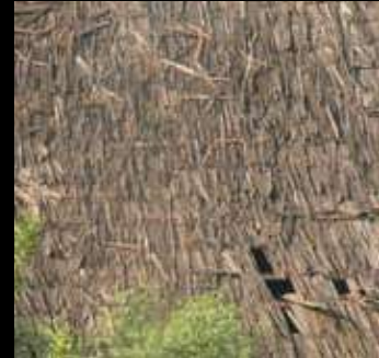
Degraded roofing with wooden shingles
