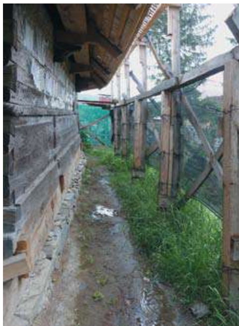
The surrounding pathway is permeable (earth) with an outer gradient that discharges rain water.
