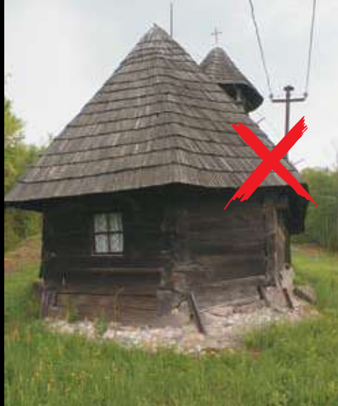
Example of common electrical connection through the roof where the shingles will deteriorate the fastest.
