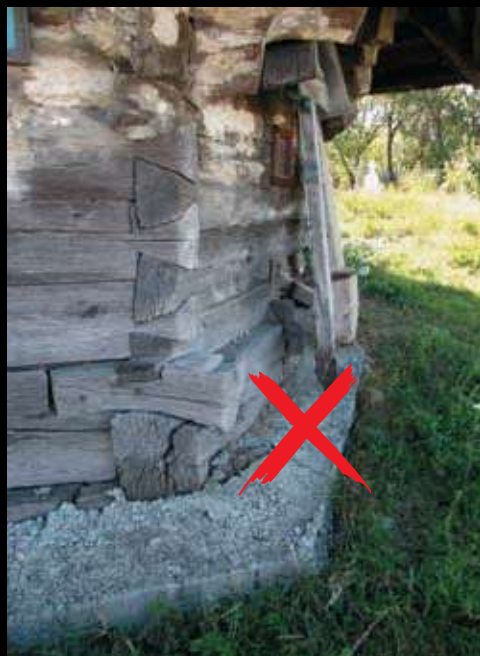
Around the church a cement layer was added that retains humidity and caused the bottom logs to rot.
