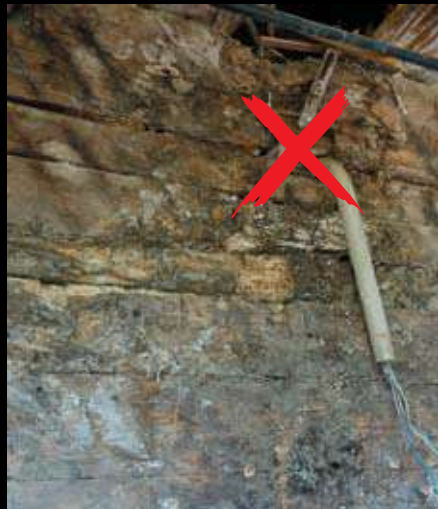
Examples of improvised electrical connections that can cause damages and can affect the church image.
