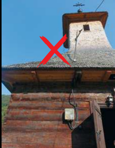
Example of external electrical connection that is not fireproof.
