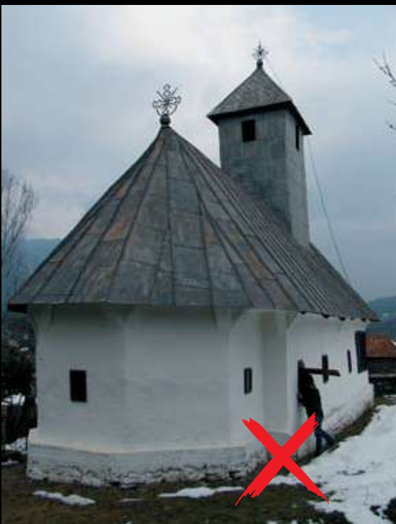
A concrete belt covering the bottom logs was placed over the stone base. This intervention is not appropriate because it will degrade the wood by rooting and weaken the structure.
