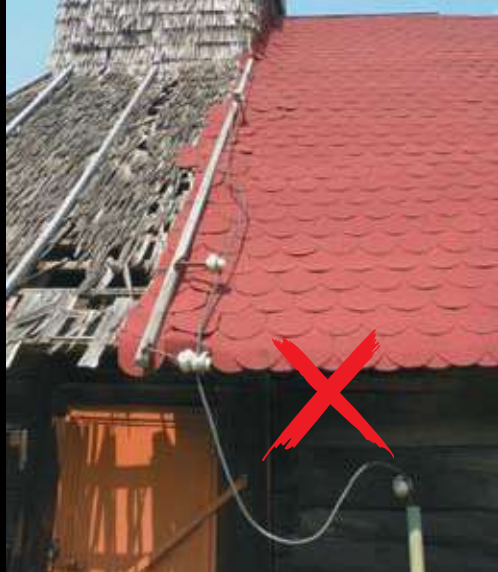
Example of lightning rod fixed on roofing in the process of replacing. Fixing spots are spots where the shingle deteriorates faster.
